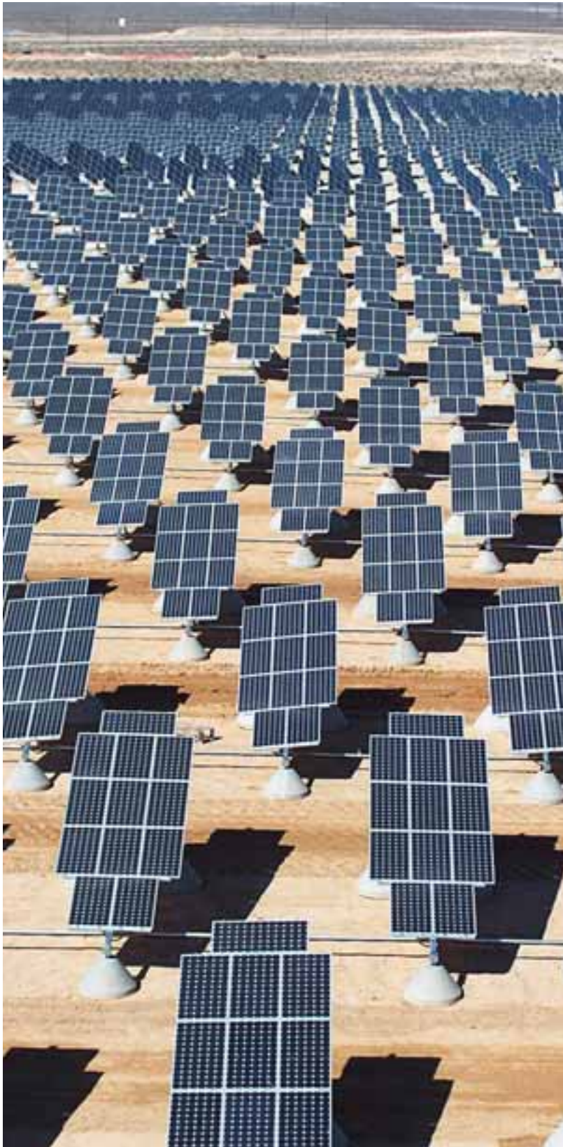
Thousands of solar panels generate electricity used at Nellis Air Force Base in Las Vegas
