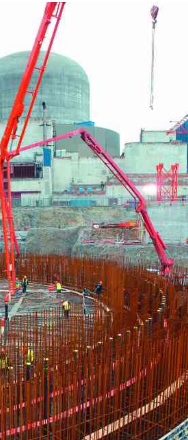
Construction site of the world's third second-generation nuclear reactor in Flamanville, northern France
