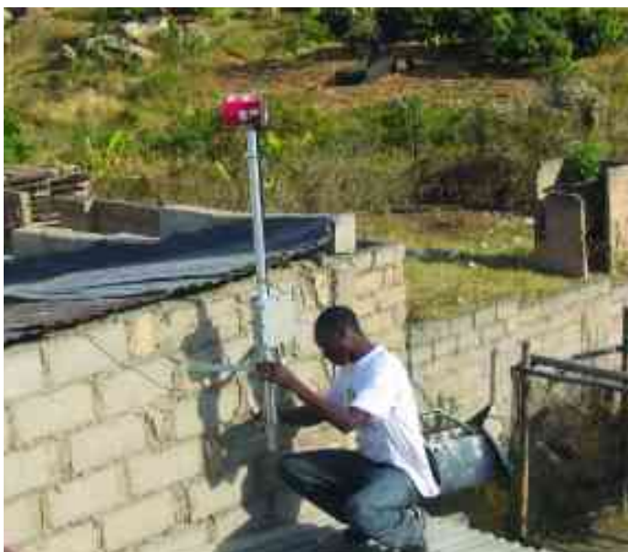
A antenna being installed on the house of a healthworker in the Peebles Valley, South Africa, connected to the HIV/AIDS clinic and other houses. A small wireless mesh network connects the hospice with an HIV/AIDS clinic and other community members, who share the cost of a single connection.
